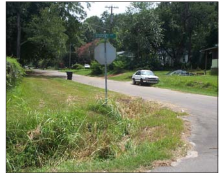
Overgrown drainage ditch at the corner of Indian River and Stuckey Street
